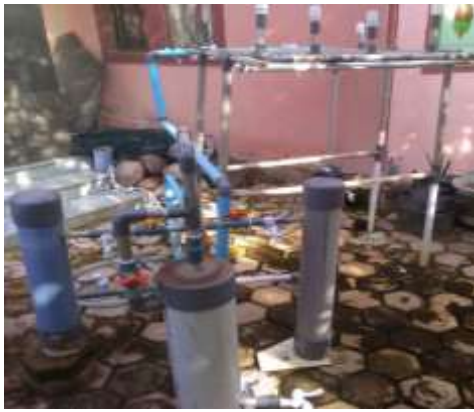
Figure 6 Unit of Fe reduction device consisting of artificial venturi, baffle, temporary deposition and filtering seen from the front
