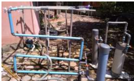
Figure 2. The unit for reducing the level of Fe which consists of a manufacturer's venturi, baffle, temporary deposition and filtering is seen from the left side
