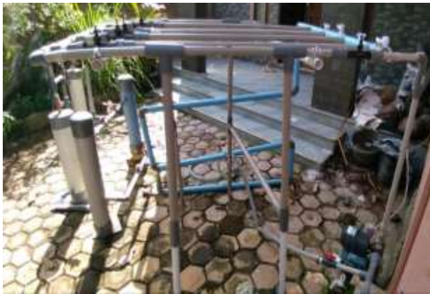
Figure 4. The unit for reducing the level of Fe which consists of a manufacturer's venturi, buffle, temporary deposition and filtering is seen on the right side
