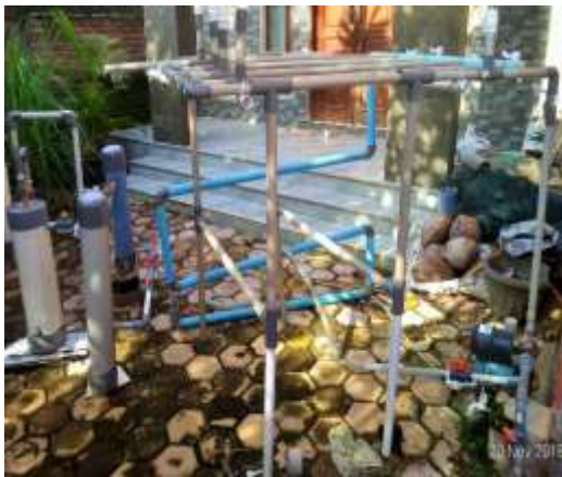
Figure 7 Unit of Fe reduction device consisting of artificial venturi, baffle pipe, temporary deposition and filtering, seen from the right side.
